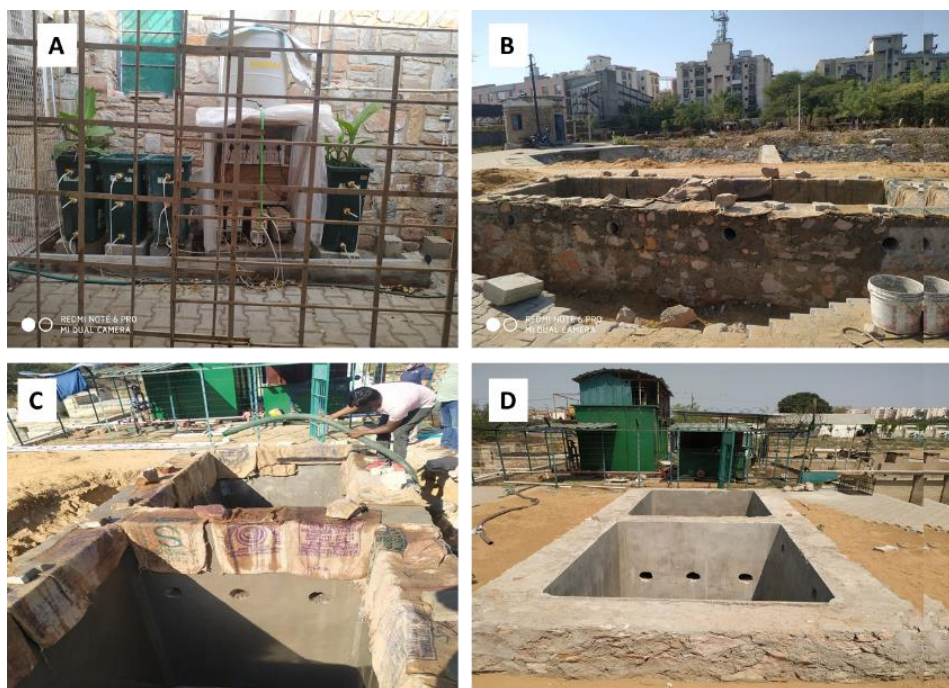
Fig. 5 Lab scale VFCW developed at MNIT (A), Progress of construction work for pilot scale VFCW at MNIT (B, C, D)
