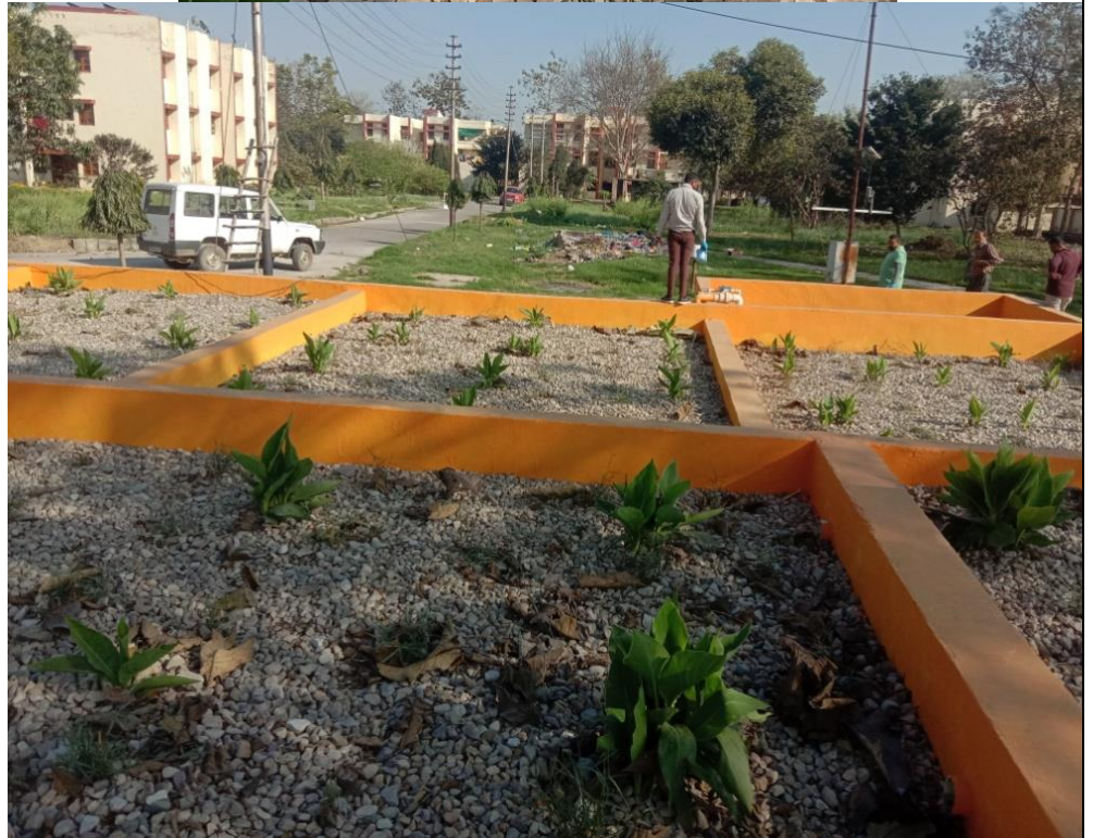
Fig. 2 Horizontal sub-surface constructed wetland (HSSCW) system in peri-urban area, Roorkee.
